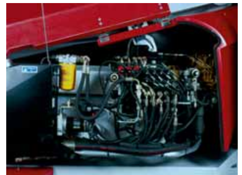
Maintenance of the modern and reliable hydraulic & control systems is easy.
